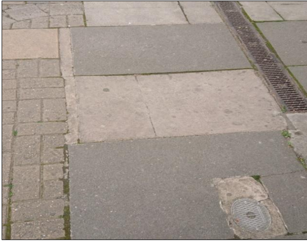
Poor paving and reinstatement, Leicester Road.
