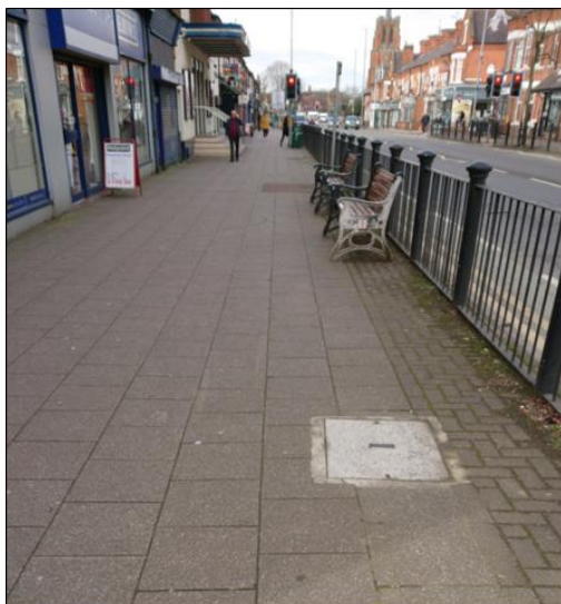
Illustration of the consistency in materials post redevelopment and shows the maintenance work needed.
