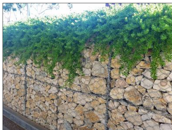
High quality example of planted stone gabions.
